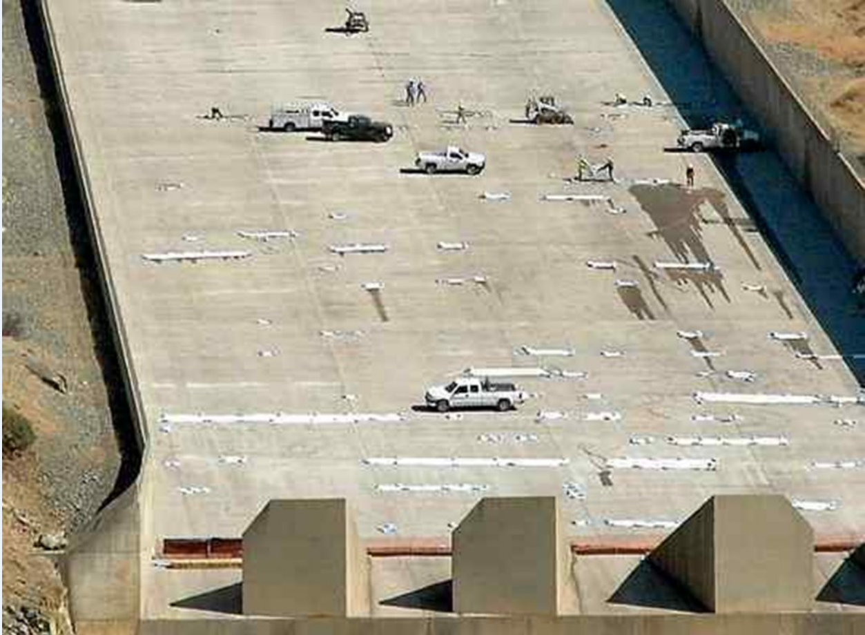
2009 Repair of Slab Cracks, Photo Cred: Barbara Arrigoni Mercury Register file photo
